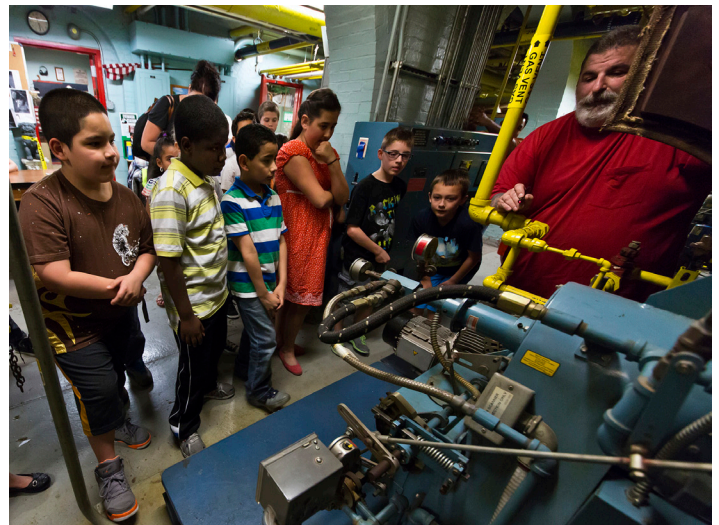
Custodian showing students how the boiler works
